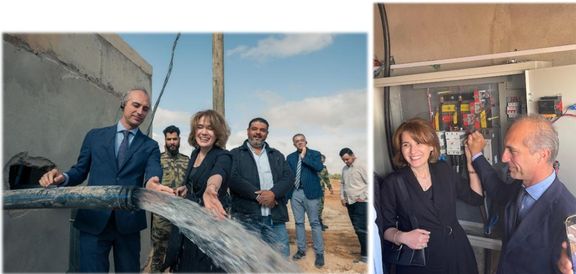
Photos 4 and 7 – Commissioning of the Awlad Yahya Pump Station during the joint verification mission to Yefren by Italian Ambassador H.E. Mr. Gianluca Alberini and UNDP Resident Representative H.E. Ms. Sophie Kemkhadze, 19 November 2025 © UNDP
