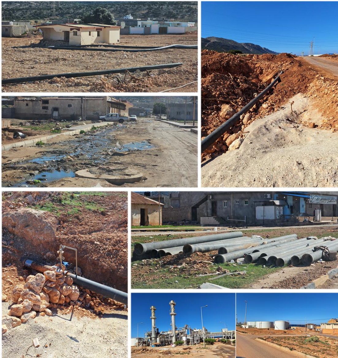
Photo 3 – Scoping the damage to water and wastewater infrastructure caused by Daniel Storm 2023 flooding © UNDP
